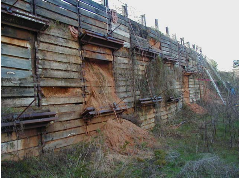
Figure 1. Tieback Wall at TAMU-NGES
