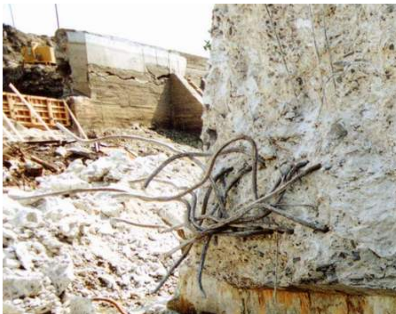
Figure 8: Exposed 100 year old rebar anchors
