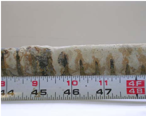
FIGURE 5. Rock Bolt # 6 With Resin Grout And Some Rust Staining Along Bonded Length.
