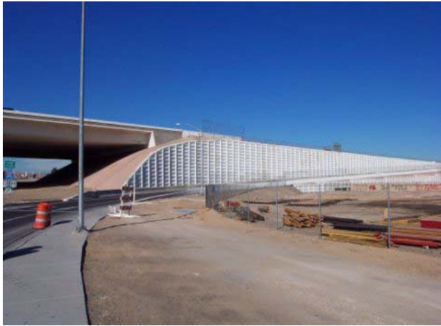
FIGURE 2(a). Wall # 1 Supporting Bridge Approach and Wall #2 Supporting On Ramp at I-515/Flamingo Rd.
