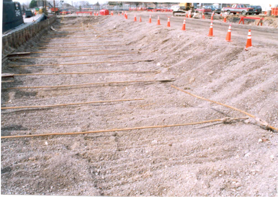
FIGURE 9 Thirty-three year old bars, backfilled in free draining gravel behind the old quay wall, and unearthed at the Buffalo Inner Harbor Project
